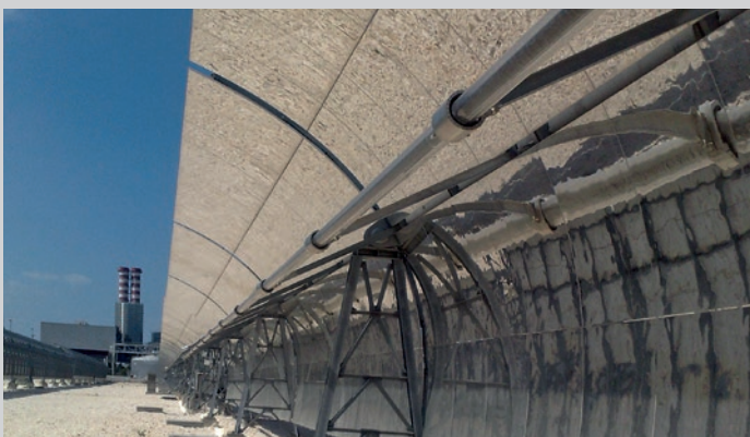
Archimede project, Syracuse, Italy A hydraulic motion system moves and controls the huge parabolic mirrors to capture the sun's rays at the solar field
